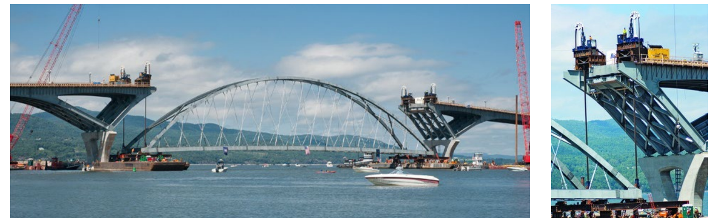
Fig. 5.11 – Lake Champlain Bridge in Crown Point, NY being lifted by hydraulic strand jacks from delta frames
