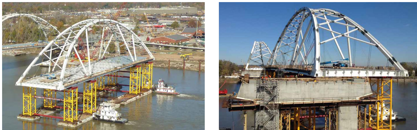
Fig. 5.9 – Broadway Bridge in Little Rock, AK being floated-in on high shoring towers from adjacent erection site
