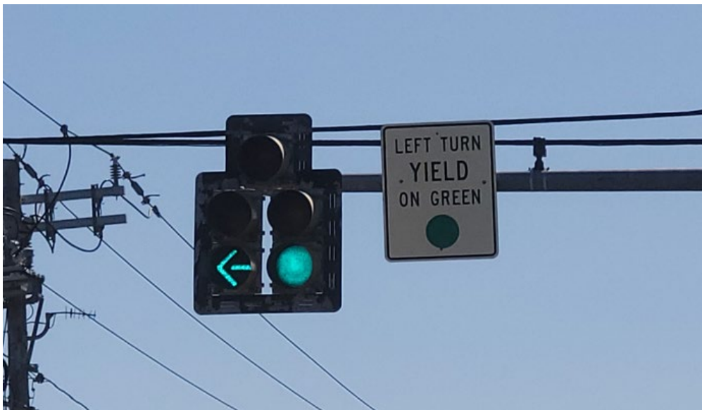
Figure 3: Traffic Signal Heads – No Retroreflective Strips on Backplates
