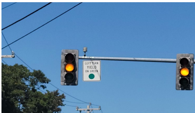
Figure 5: Pleasant Lake Avenue (Route 124) Southbound Approach Left-Turn Signal Head - Circle Green Indication
