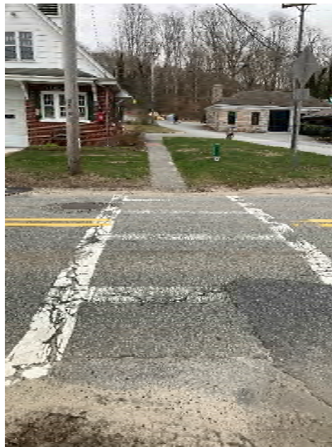
Image 6: Crosswalk with Faded Striping on Route 28A at the Falmouth Fire Department Station 4
