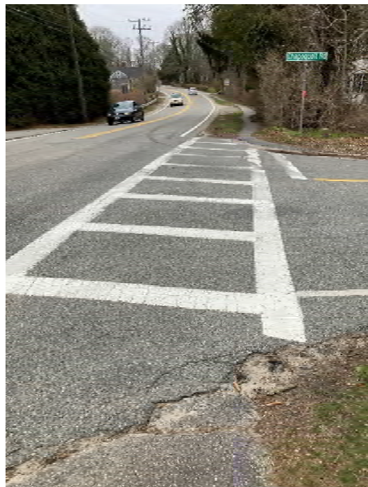
Image 9: Crosswalk at Chapoquoit Road Does Not Have Accessible Curb Ramps
