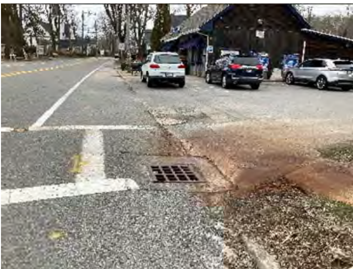
Image 8: Crosswalk at the West Falmouth Market with a Catch Basin in the Path of Travel
