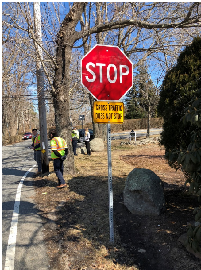
Figure 12 – Mary Dunn Road stop sign with warning plaque
