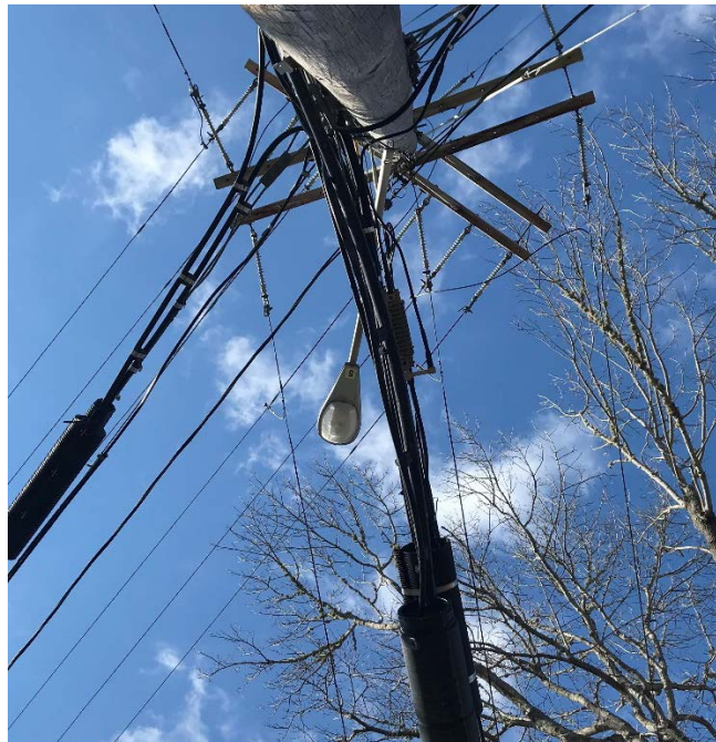
Figure 9 – Existing Street Light
