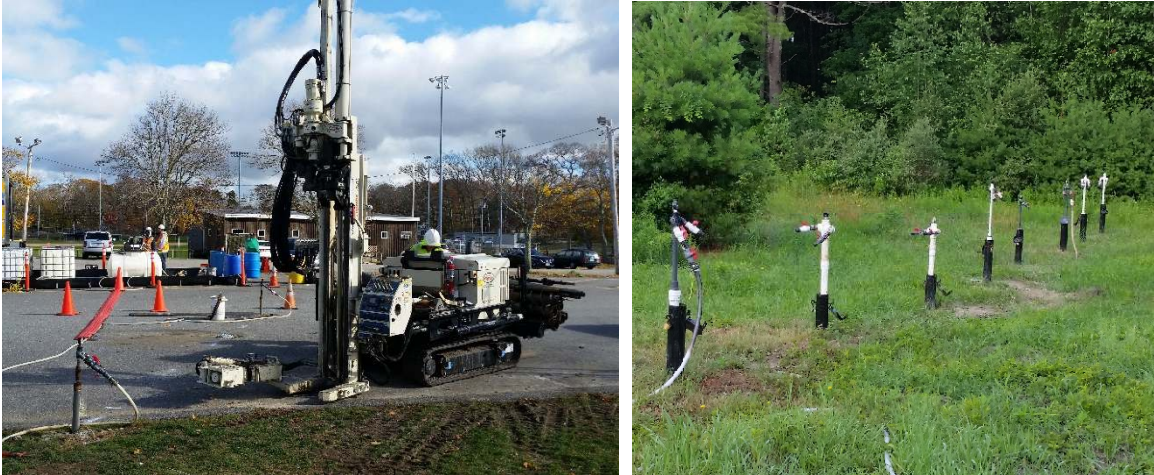
Figure 4. Direct-push drill rig used to advance temporary injection points for a PRB, and injection PRB using PVC injection wells.
