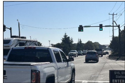
Image 2: Signal head have LEDs burned out and are missing retroreflective backplates.
