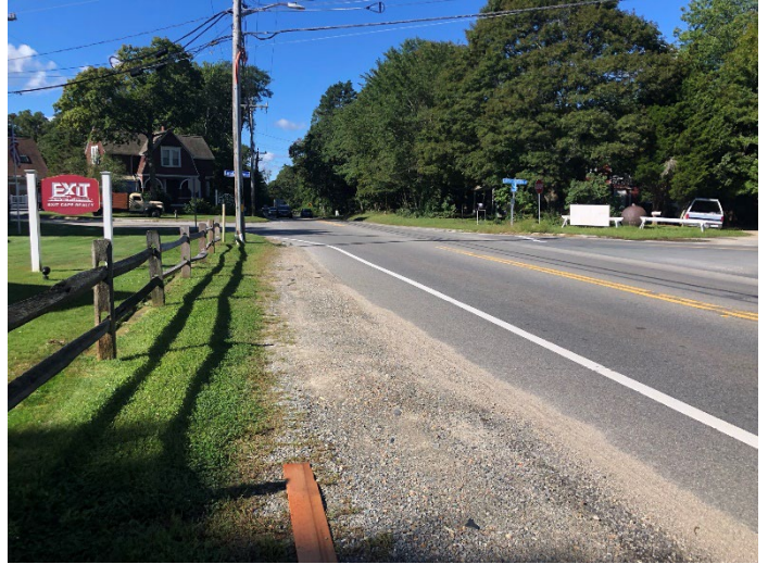
Image 7: A View looking westward toward the intersection. Bus pullout for eastbound buses is in foreground. Note the lack of bicycle and pedestrian accommodations (except for shoulders)
