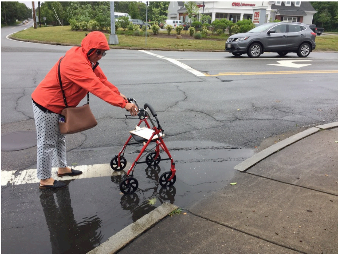
Ponding at curb ramps impede access.
