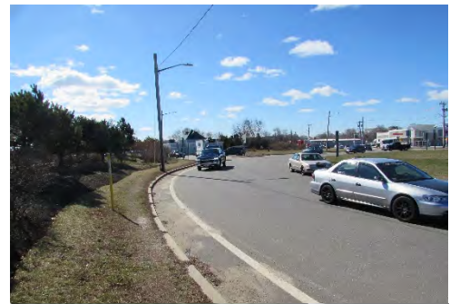
Image 1: Lack of Lane Definition within Barnstable Airport Rotary
