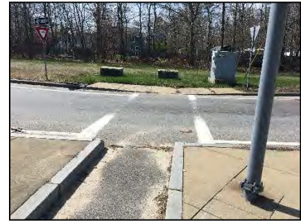
Image 7: Lack of yield markings on northbound right turn
