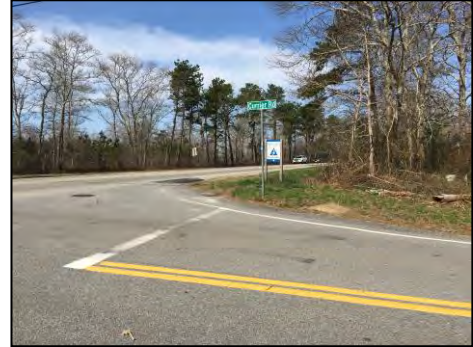
Image 3: Faded stop bar and missing stop sign on Southbound Currier Road
