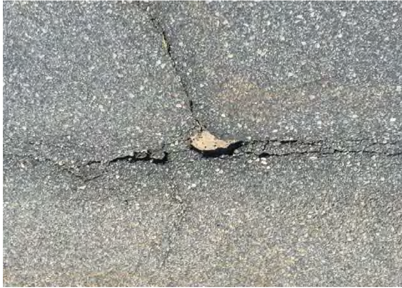
Figure 11 - Example of pavement distress
