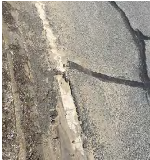
Figure 6 - Edge line markings obscured by sand
