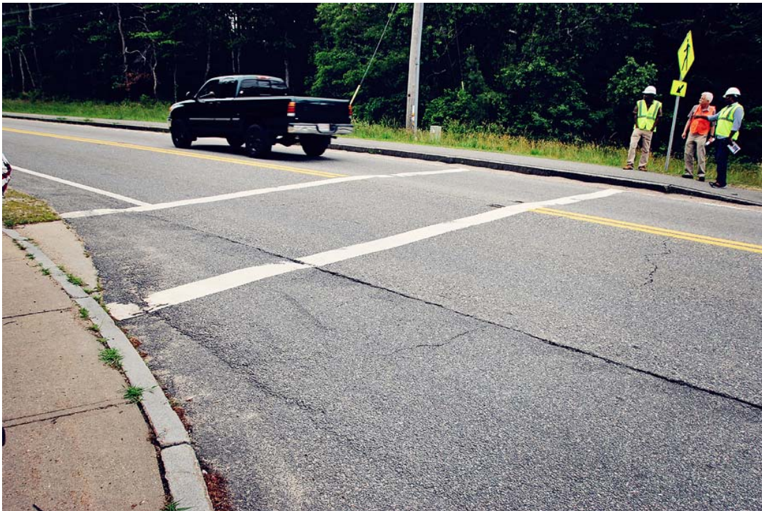
Figure 7 - View looking southbound of the pedestrian crosswalk crossing Route 132 depicting no accessible ramp for pedestrians on the opposite side of the street
