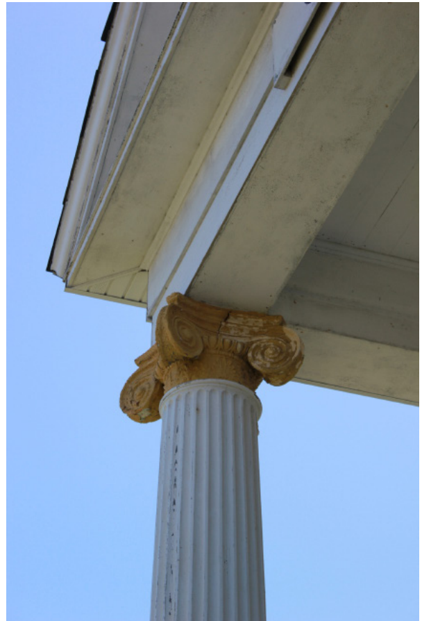
Detail of column. A crack can be seen at the capital.
