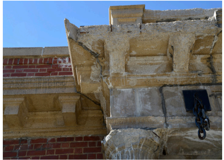
Large pieces of concrete have crumbled and fallen off the building
