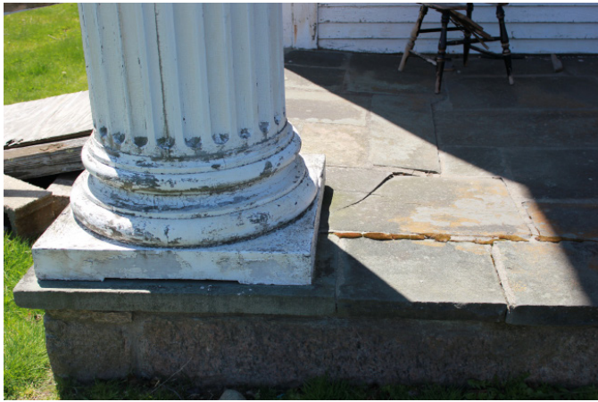
Detail of column base and porch. A crack can be seen on the porch.
