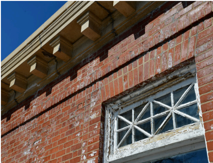
Efflorescence and spalling are signs of excessive moisture
