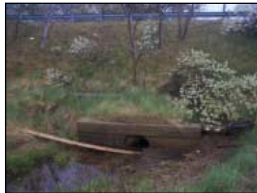
This 2-foot diameter concrete culvert passes tidal flow under Route 6, but it first must pass through the seaward channel that is clogged with dead grasses.
