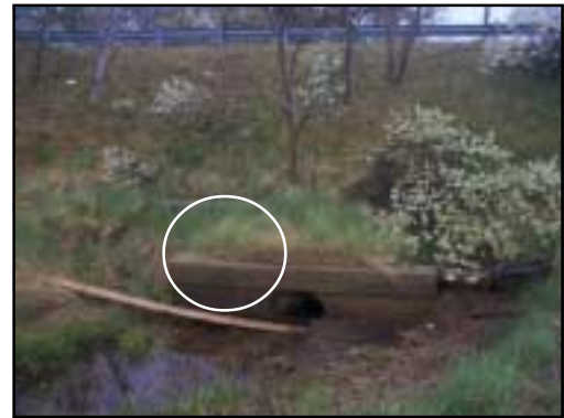
A large quantity of debris has collected near this seaward headwall and partially blocks the pipe, which is submerged beneath the brown murky water and located just to the left of a Route 6 drainage pipe (clearly visible here to the right of the stone headwall).
