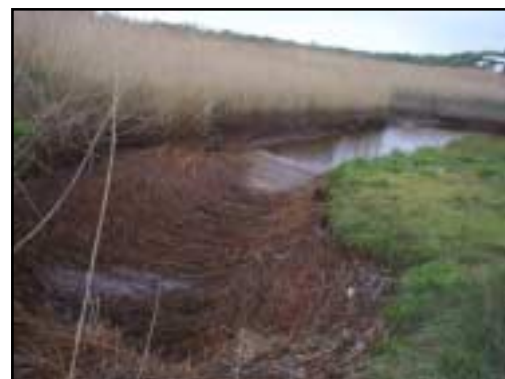
Phragmites dominates the upstream affected area. Dead reeds and debris have collected near the upstream opening, obscuring the pipe from view.
