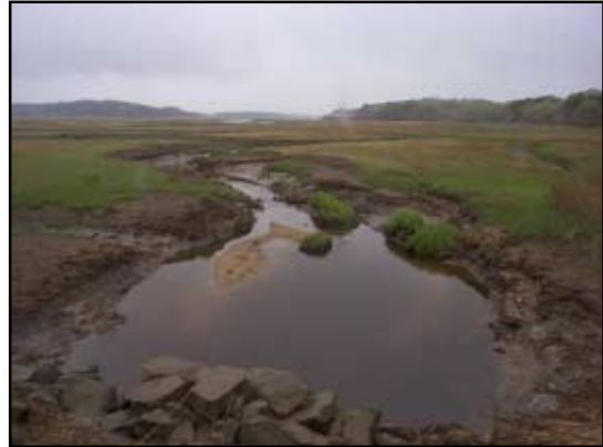
Looking from the culvert into the seaward salt marsh area several visual indicators of a restriction dominate the view, including vegetation die off, scouring, erosion, and marsh slumping.
