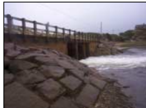
These 3 box culverts viewed from the seaward side of Chequessett Neck Road, two fitted with flapper gates and one with a sluice gate, control the exchange of salt and fresh water between the Herring River and Wellfleet Harbor.
