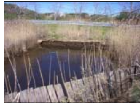
The 3-foot metal pipe and clapper gate set within this headwall (visible below the water line) pass only the seaward flow of the Pamet River under Wilder Dike (Truro Center Road/Route 6A).
