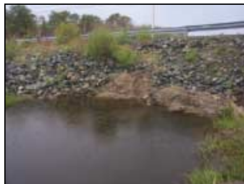
The berm of Old County Road partially dams Eagle Neck Creek. The upstream pipe is visible in this pool and is blocked by rocks – further restricting tidal flow.
