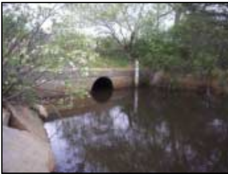
After crossing underground for approximately 375 feet the Pamet River emerges upstream of Route 6 through this 4-foot opening in the concrete headwall.
