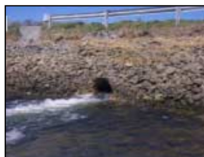
This 3-foot culvert passes tidal flow under Mill Pond Road, here water is seen rushing seaward on an outgoing tide.
