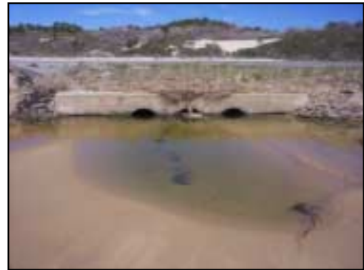
A large scour pool is visible in front of these three 30-inch culverts. Water marks and debris left by high water are visible on top of this headwall.
