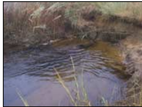
The seaward side of the berm is subject to severe scouring and erosion. The submerged 1-foot clay pipe is seen here during an outgoing, low tide cycle.
