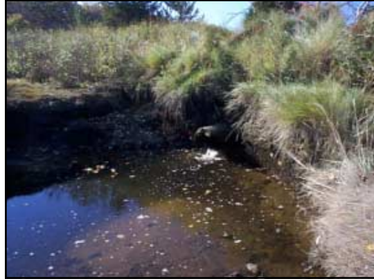
A culvert invert problem observed in Sandwich, at site SA-11 – the pipe is sited high in the bank; too high to pass the full tidal range.
