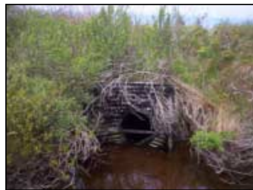
This corrugated metal sluiceway is located on the upstream side of the dike, with its opening approximately 1-foot lower than the seaward side's opening.
