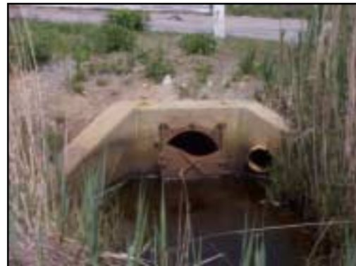
This broken clapper gate covers the 30 inch pipe and restricts the incoming tide under Governor Prence Road.
