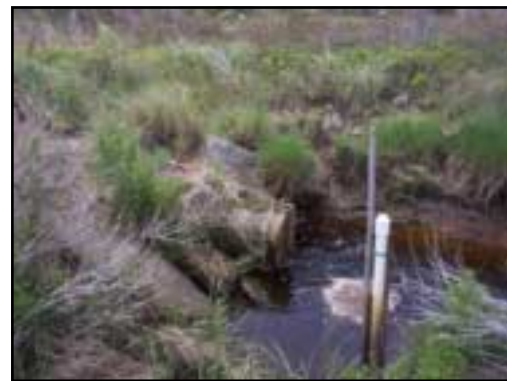
This flapper gate prevents tidal flow from passing upstream via the 2-foot pipe. Note the tide gauge installed at this location.
