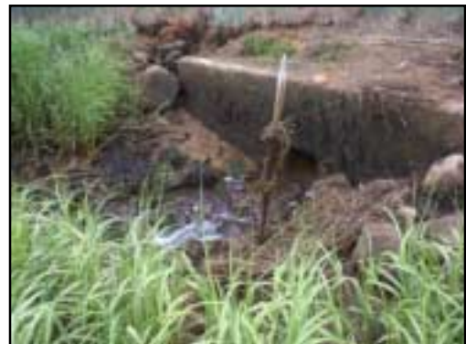
Scouring and erosion scar the upstream side. As was the seaward headwall, this side is consistently submerged. Note the placement of the tide gauge to monitor flow in this system.
