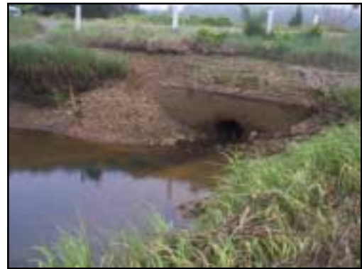
The roadway berm around this seaward headwall and the channel edges are severely eroded. A wide, deep scour pool has formed in front of this 28-inch opening.
