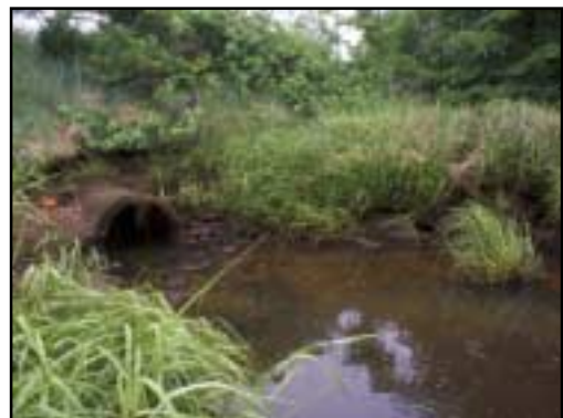
Upstream of the bike trail the bank has eroded away from this 36-inch pipe. Scour and erosion scar the area.
