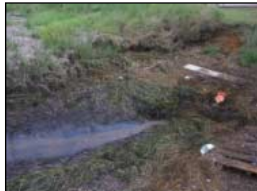
Water trickling out of a mound of dead seaweed near the seaward opening enabled field staff to dig out the opening of the 10-inch pipe. Erosion is a serious problem near the opening.
