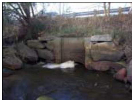
The seaward opening is nearly submerged even well before the tide is high. Watermarks are visible near the top of the headwall.
