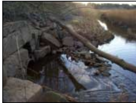
This headwall supporting the upstream opening is in need of repair—it is eroding and falling into the channel below.
