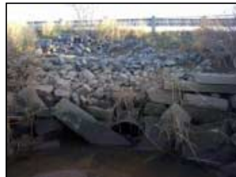
The seaward culvert is visible at low tide with water pooling by this partially blocked opening.
