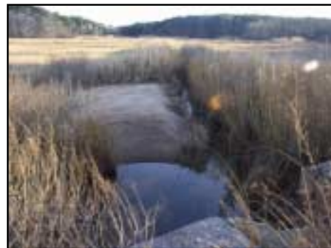
A large sandbar has formed in the upstream channel near the culverts' scour basin – road runoff from the nearby major road junction is a likely source.
